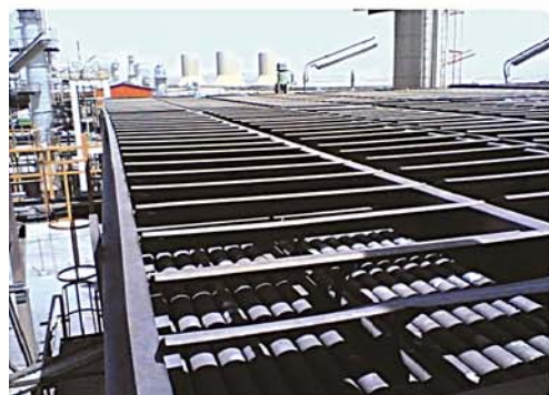
Louver Isfahan Oil Refining Co.
